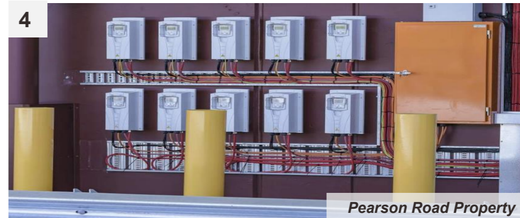
Electricity and water sub-metering to allow for monitoring, management and reporting of building performance
