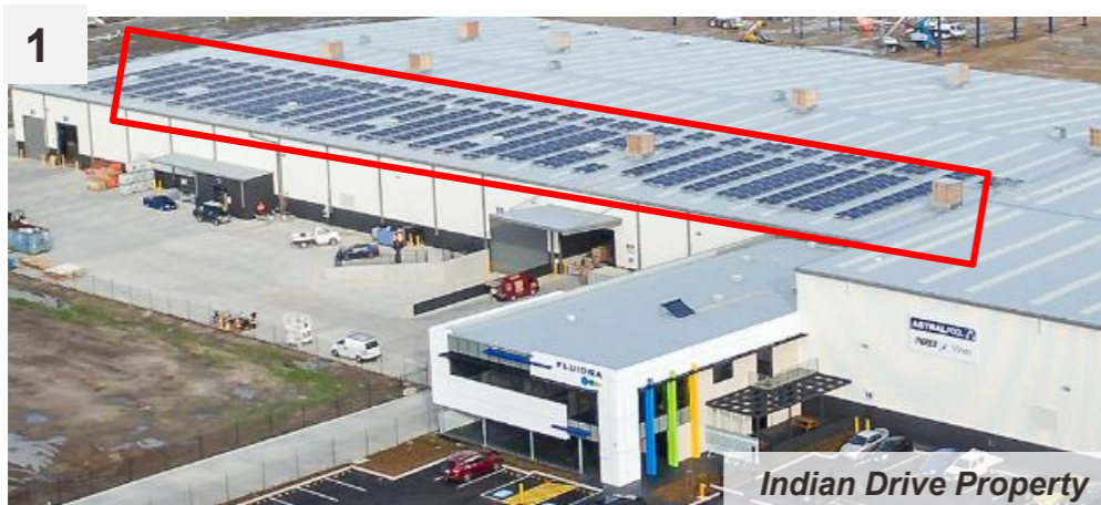
Solar PV system to generate renewable energy for use on site
